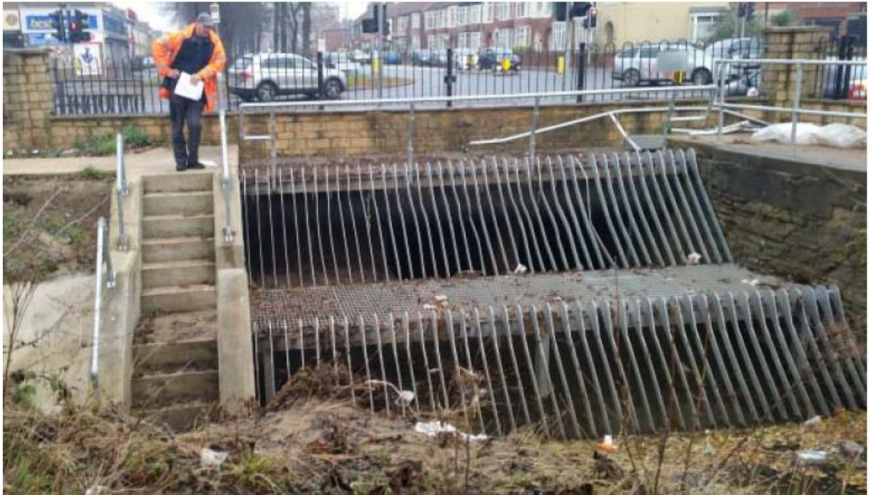
Albert Park Trash Screen day after near flood
